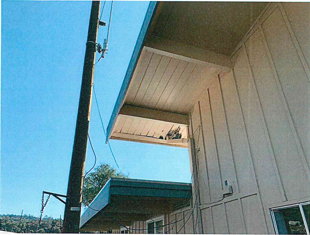
Photo 3 severe rot needs replaced in-kind at re-roof.
